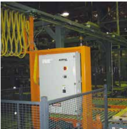
PCV linear feedback ensures material handling system transfer cars allocate their pallets to the correct conveyor.
